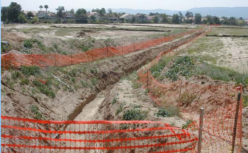
Land developer straightened and filled channel without 401 Certification
